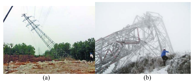
Figure 1: Tilted and collapsed tower
